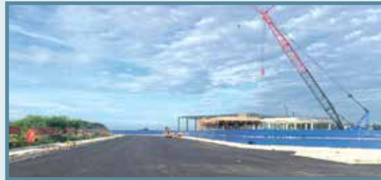
Logistics Hub Infrastructure
