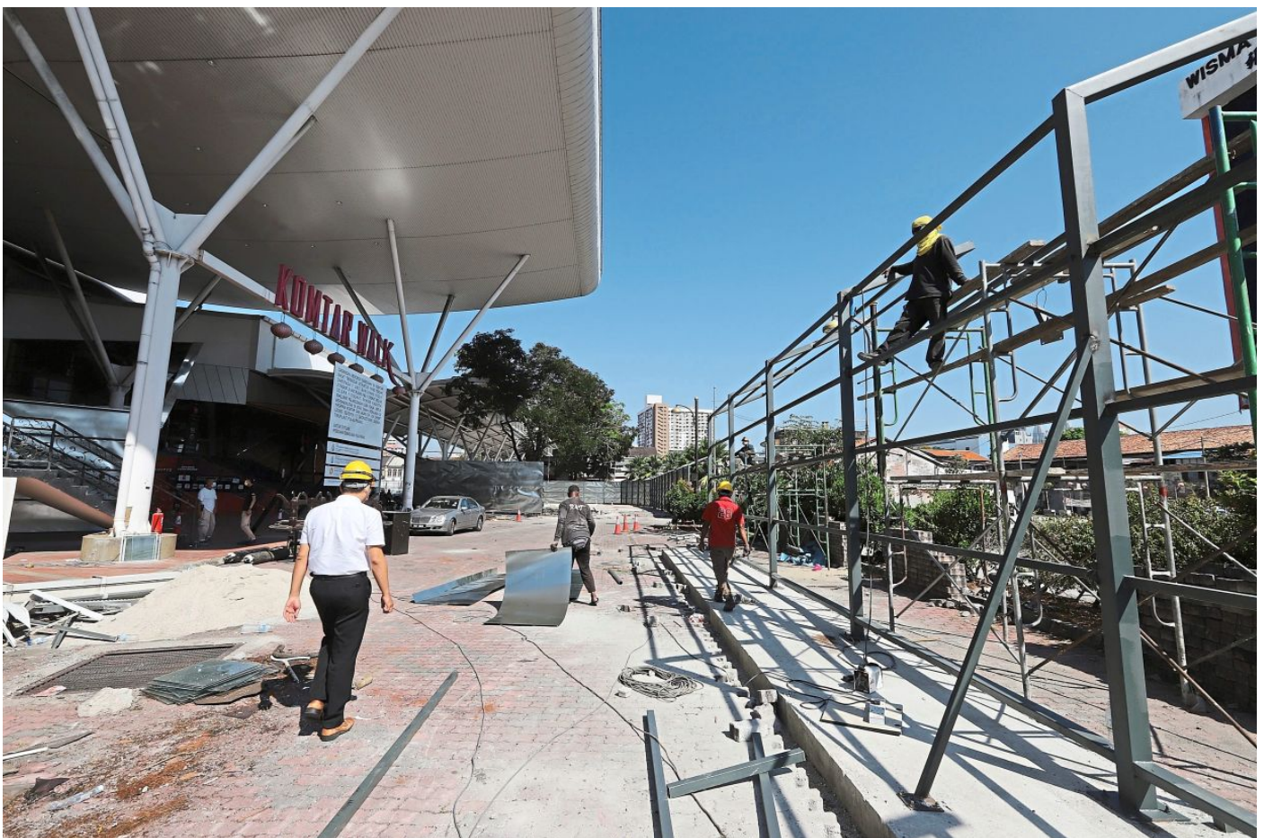
Demolition work in progress at the entrance of Komtar Walk beside Jalan Dr Lim Chwee Leong in Penang.
